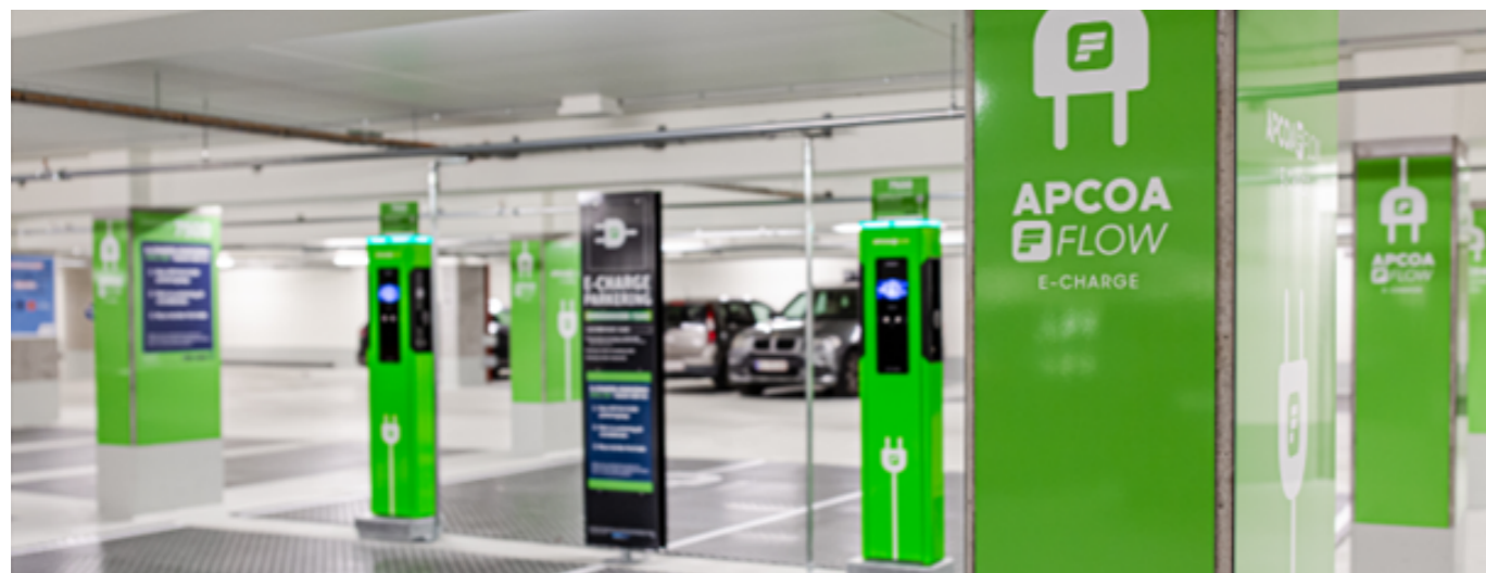
Fig. 18: APCOA Parking Denmark (2022), EV Charging
